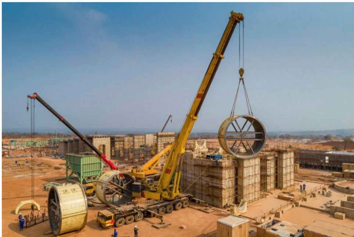
The Kamoia-Kakula mine under construction. The site was one of the largest discoveries in the history of the African copper belt © Ivanhoe Mines
